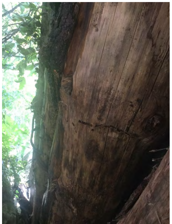
Stringer 12 - cracked midspan
